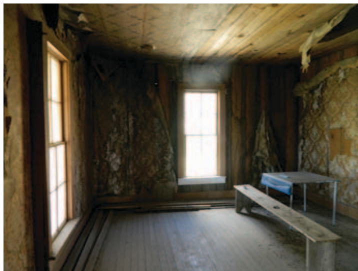
Fig. Parlor_5: Extra siding stored on floor; debris accumulating on floor.
