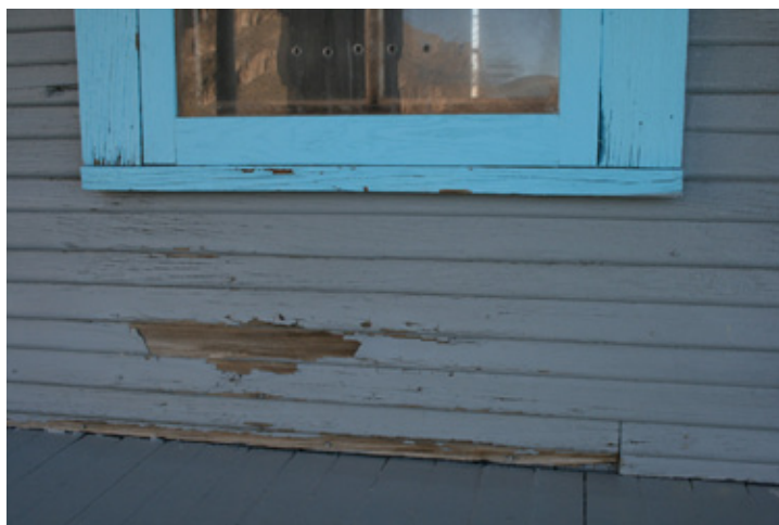
Fig. Exterior Cladding_6: Chipped and flaking paint on the siding.
