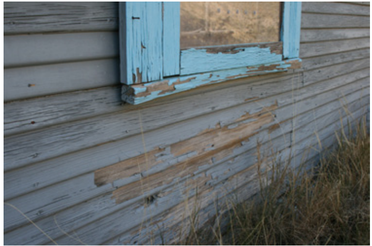
Fig. Windows and Doors_1: South window on eastern elevation has warped sill and peeling paint.
