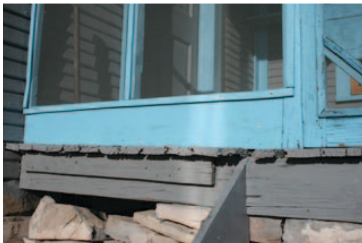
Fig. West Porch_3: Porch floor uneven. Floor boards warped with some deterioration on the exterior ends; note warped end of screen frame in lower left corner
