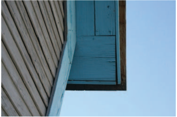
Fig. Roof_4: Eave separating at northeast corner of house.
