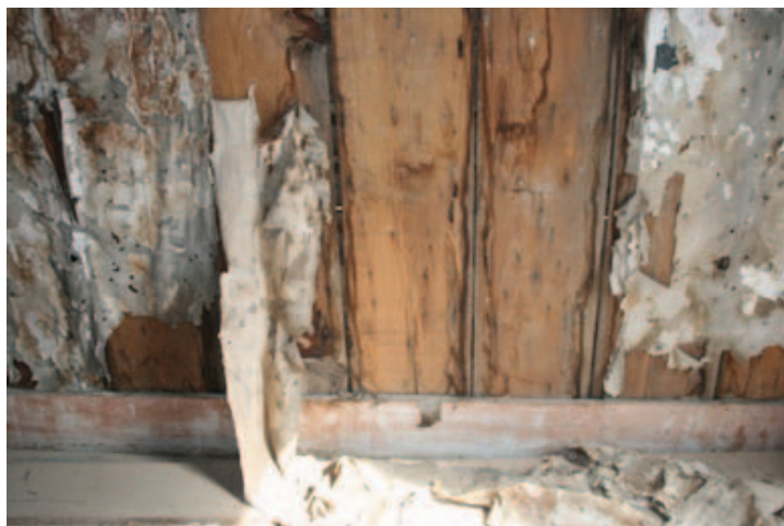
Fig. Kitchen_3: Fallen wallpaper on east wall; white residue on baseboard; deterioration of baseboard.
