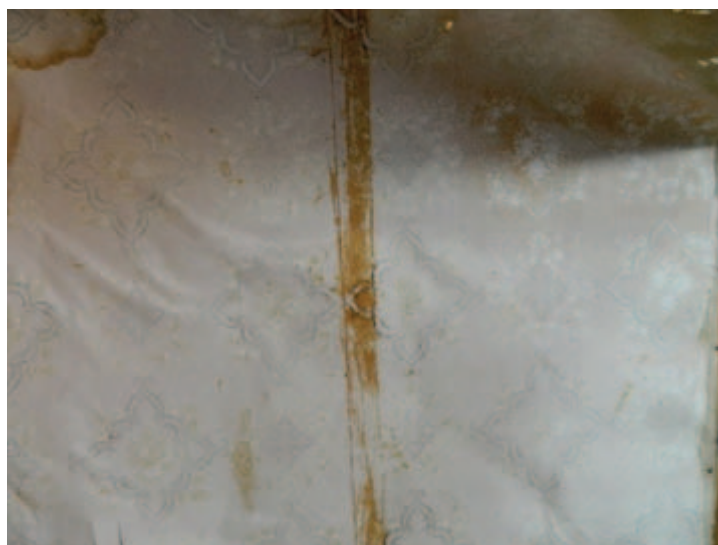
Fig. Bedroom_2: Remaining wallpaper on ceiling faded and stained.
