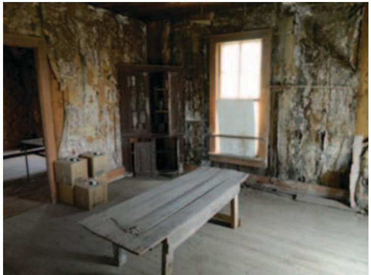
Fig. Kitchen_2: Kitchen facing northeast; note water staining and detachment of wallpaper.
