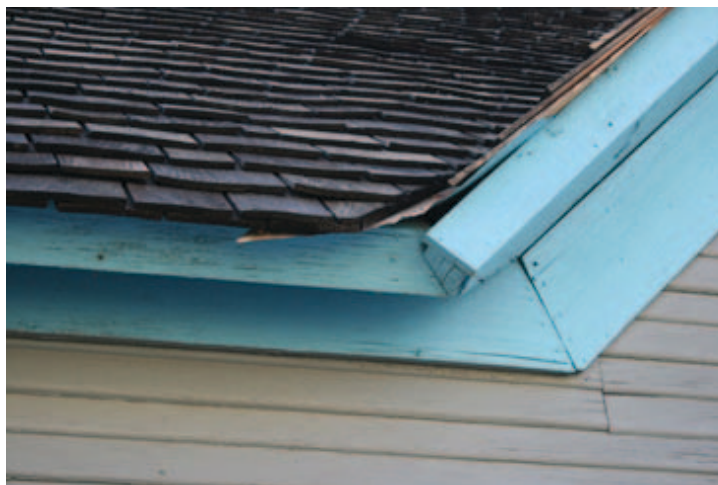
Fig. Roof_1: Protruding flashing and nails at eave on east façade. Note that the corners of the trim and eave do not line up.
