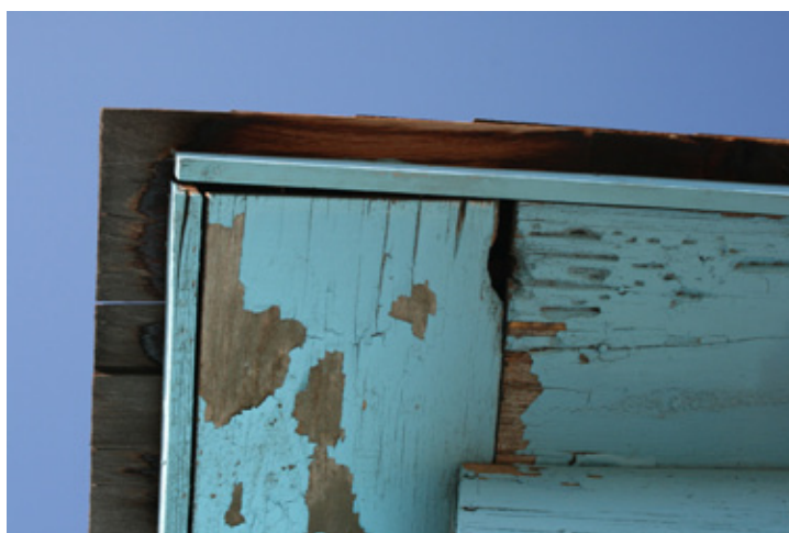
Fig. Roof_3: Paint peeling on soffit at the southwest corner of the house; note separation of eave.
