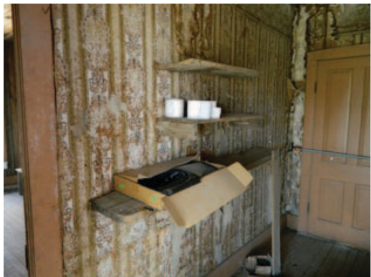
Fig. Foyer_2: Foyer shelves, facing southeast; note debris on floor.
