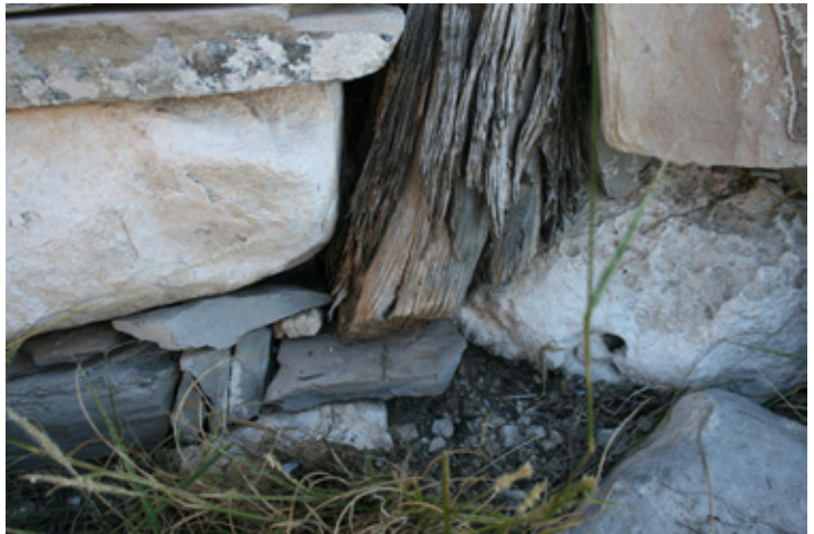
Fig. Foundation/Crawl Space_2: Post under north porch too short. Replacement will require moving and resetting foundation stones to accommodate burying post below grade.
