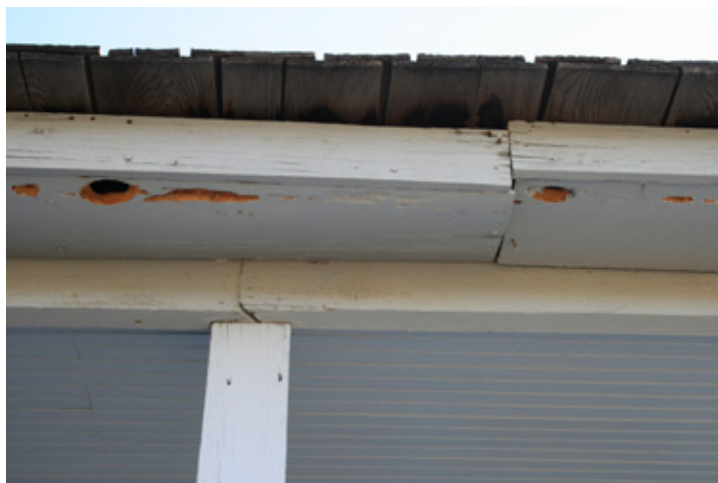
Fig. North Porch_2: Separation of butt joints near center post on north porch. Woodpecker damage to soffit.
