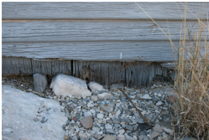
Fig. Exterior Cladding_1: Missing siding on east side of house. Note that the interior vertical planks are resting directly on the ground (should be monitored for deterioration).
