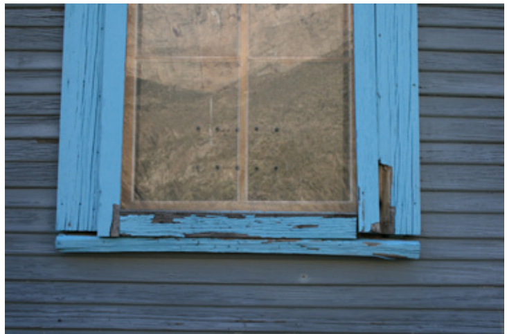
Fig. Windows and Doors_2: North window on eastern elevation exhibits slippage of the sill and cracking of the frame.
