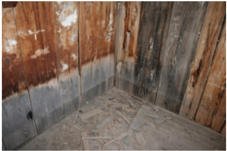
Fig. Pantry/Washroom_5: Water staining and splash line on vertical planks in south and east walls; it is possible that this resulted from use of the room.
