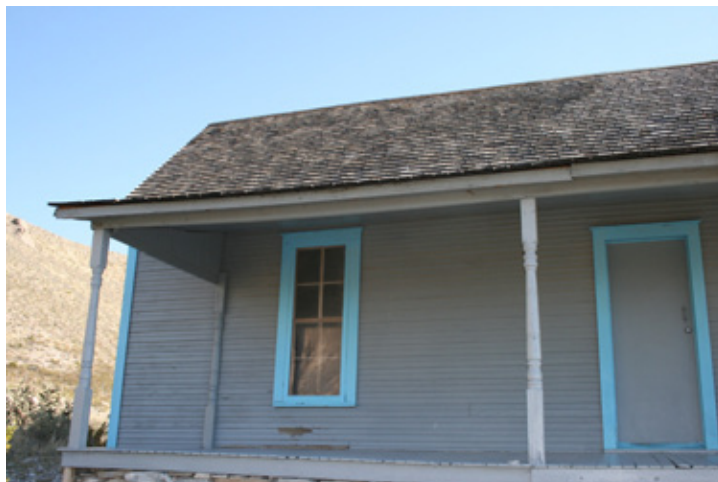
Fig. North Porch_1: Northeast section of fascia sagging, may indicate movement.
