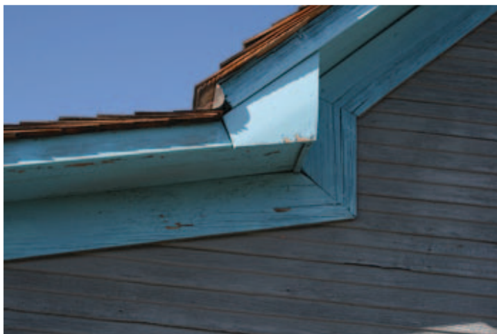
Fig. West Porch_4: Hip joint of shed roof over west porch and interior storage room and main gabled roof is not very tight; may allow water to enter.
