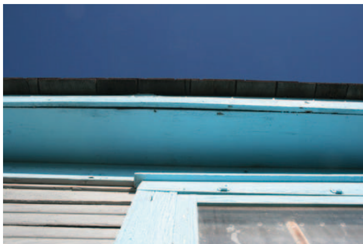
Fig. Roof_2: Fascia board warped on west façade.
