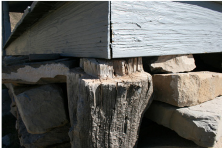
Fig. Foundation/Crawl Space_1: Post not seated properly under northwest corner of north porch.
