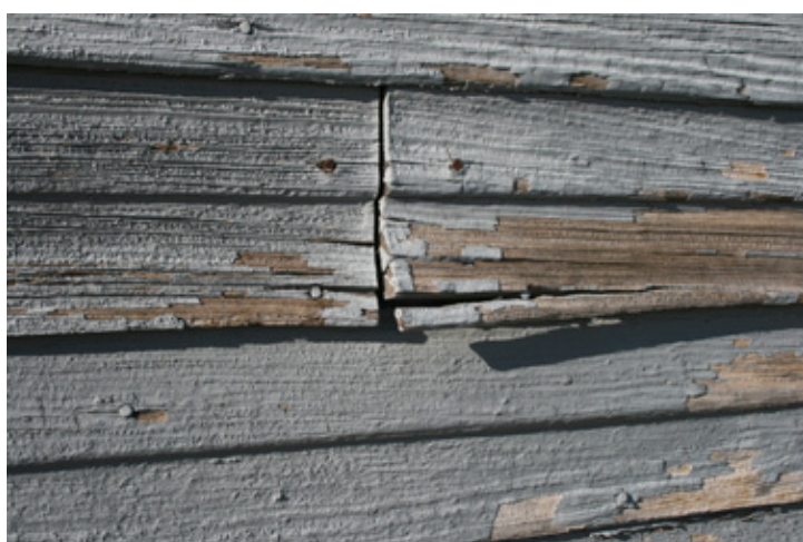
Fig. Exterior Cladding_3: Deterioration of siding in places includes cracking, splitting, and UV degradation.
