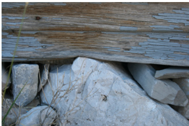
Fig. Exterior Cladding_2: Slight settling has caused deformation of siding at the base of the easter wall.
