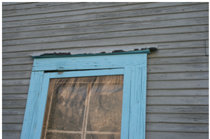
Fig. Windows and Doors_3: North window on eastern elevation shows wear to the flashing and sash has slipped.
