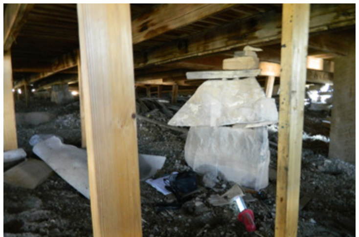
Fig. Foundation/Crawl Space_8: Evidence of pests (pack rat).
