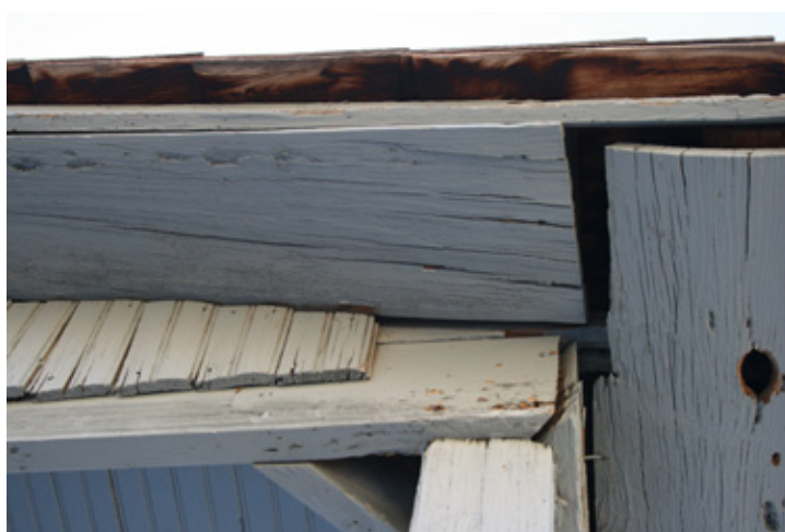
Fig. North Porch_3: Separation of soffit at northeast corner of porch due to warping of board. Note missing piece of decorative beadboard.
