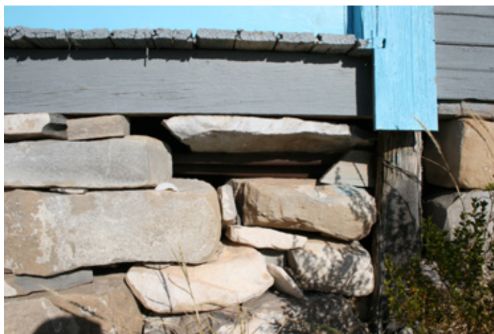
Fig. Foundation/Crawl Space_5: Missing foundation stones.
