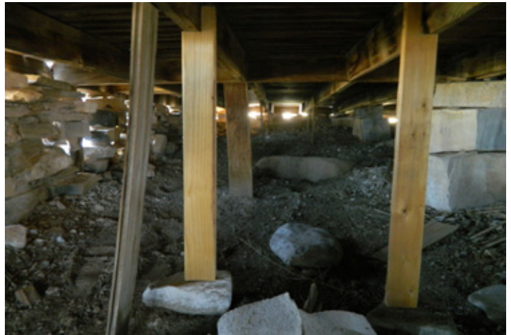
Fig. Foundation/Crawl Space_7: Varied shoring under floor joists.
