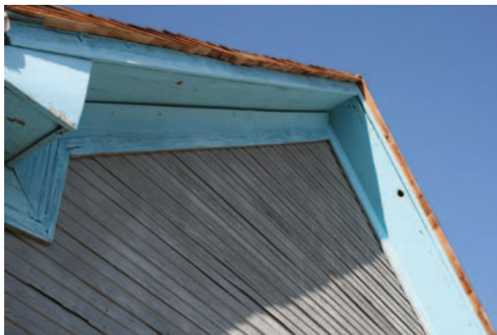
Fig. Roof_6: Trim warped at gable on south façade.
