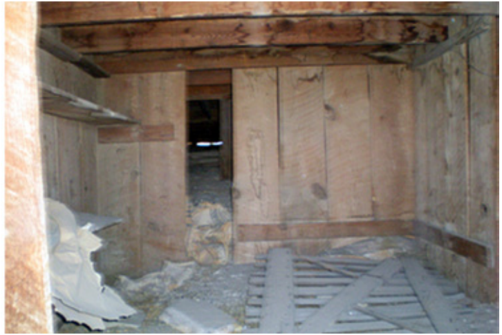
Fig. Foundation/Crawl Space_6: Debris, some historic, in crawl space.
