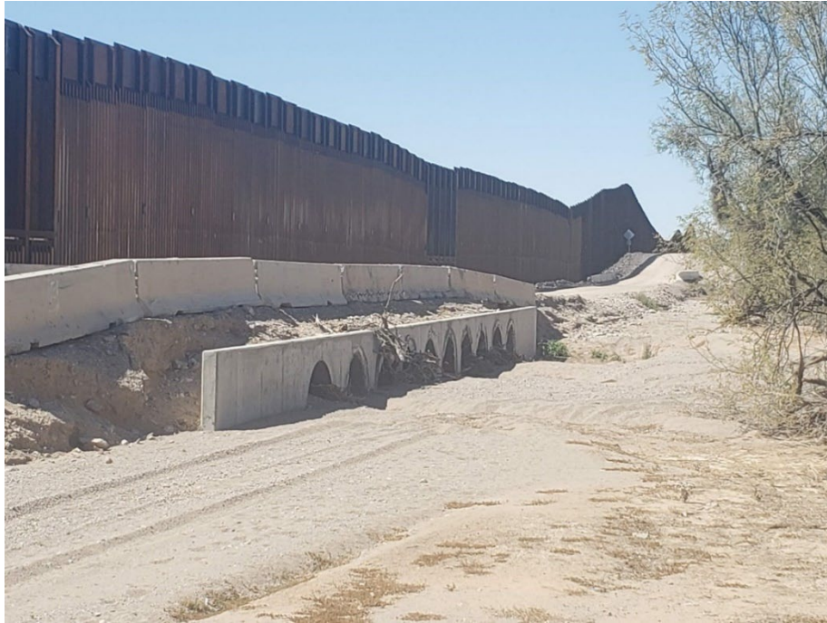
Figure 5-22 Drainage at southern end of Aguajita Wash adjacent to Aguajita Spring (Nov. 2022). Teresa DeKoker, photographer
