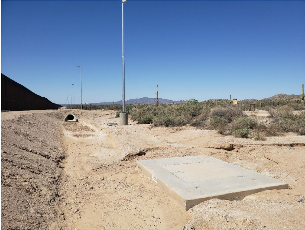
Figure 3-51 Drainage ditch placed with border wall construction in 2020, facing west (Nov. 2021) Teresa DeKoker, photographer
