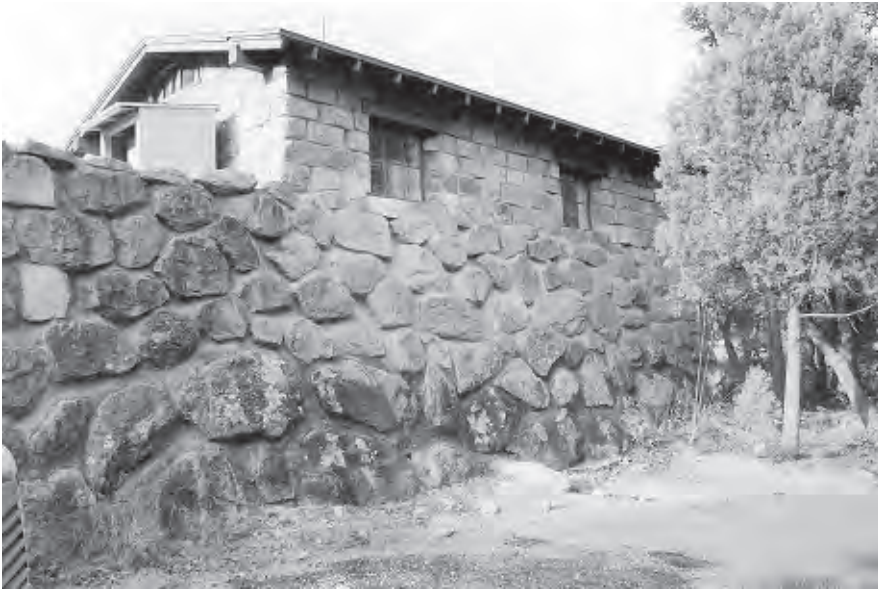
Figure 125. The Power House and Laundry incorporates the utility wall as part of its north and west faces, 2002. View looking southwest.
