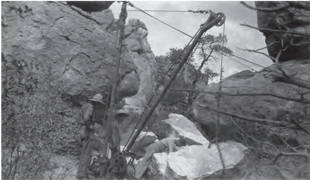
Figure 22. Trail crews used a portable hoist system with boom and winch to move large rocks.
