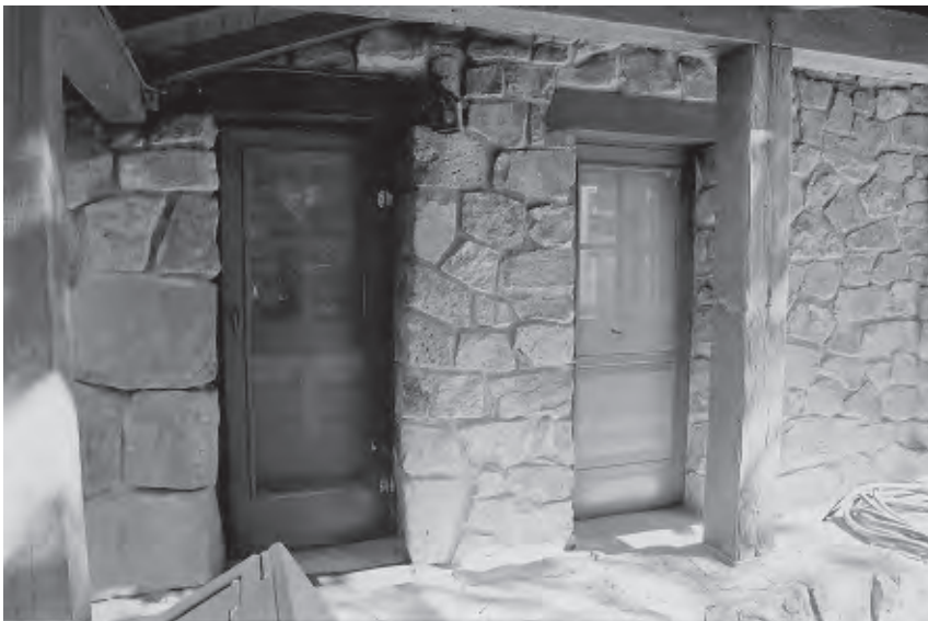
Figure 79. Additional door on right was added in 1965 to rear of Administration Building, 2002.
