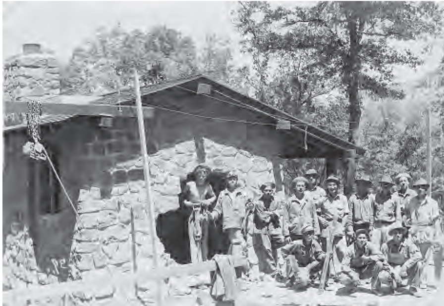
Figure 74. CCC enrollees create opening in Ranger Station to accommodate east wing of Administration Building, 1937. Note excavation for basement on left. View looking northwest.
