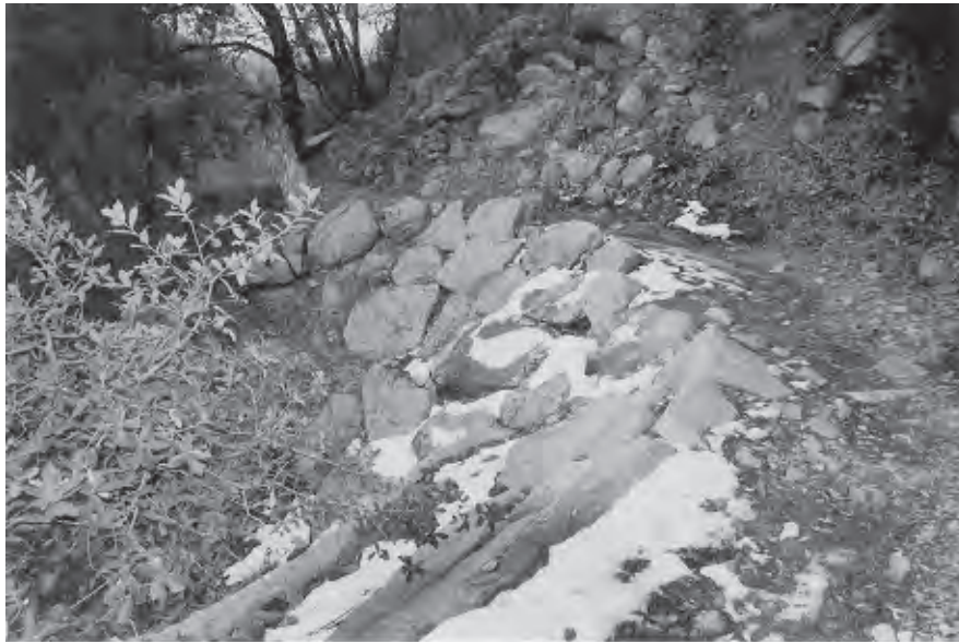
Figure 24. Retaining walls on Lower Rhyolite Trail show damage from rainstorms, 2002.
