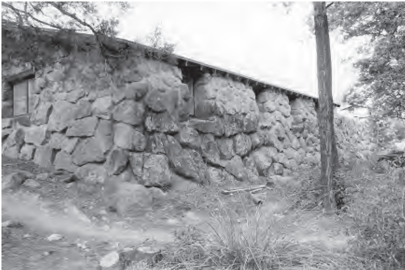
Figure 117. Northeast corner of the utility wall is constructed with largely uncut, uncoursed boulders, 2002. The wall is strongly battered. Note Warehouse incorporates wall in east and north faces. View looking southwest.
