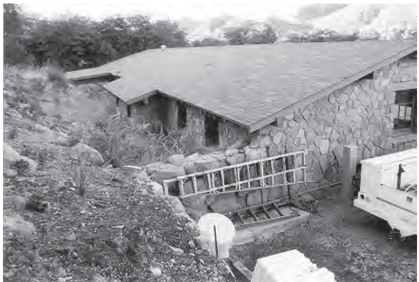
Figure 118. The Southeast retaining wall was added on to existing Equipment Shed, 2003. Note difference in stonemasonry of the Equipment Shed and adjoining utility wall. View looking northwest.
