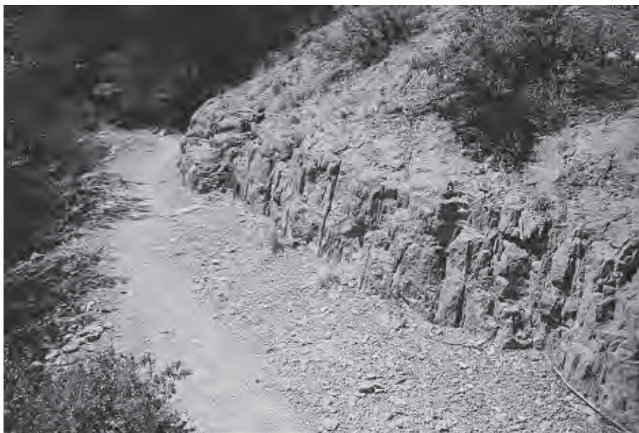
Figure 23. Evidence of drill work in upper slope cuts on Lower Rhyolite Trail.
