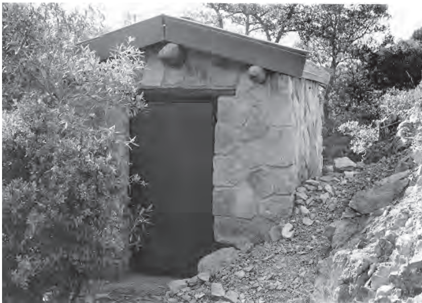
Figure 86. Second Cap Magazine with steel door, vigas, and replaced roof, 2003. View looking west.
