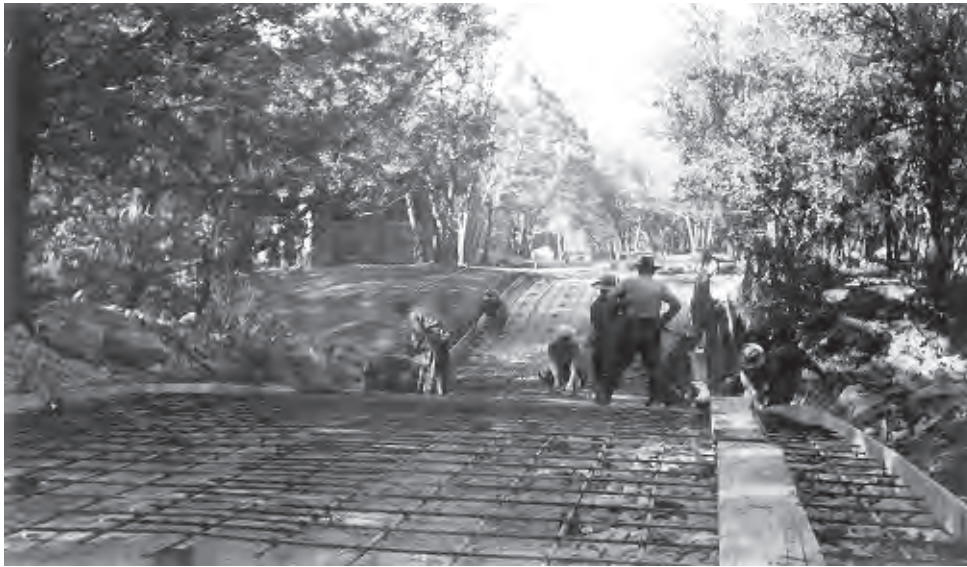
Figure 87. CCC enrollees lay wire mesh prior to pouring concrete in first campground "dip," 1935. View looking southwest.
