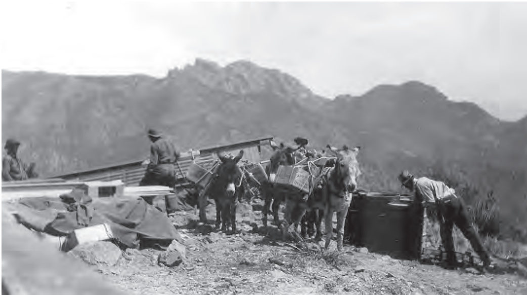
Figure 105. CCC enrollees used mules to haul materials to Sugarloaf Mountain during construction of the Lookout, 1935. Note boxes of dynamite for excavating the Lookout foundation. View looking north
