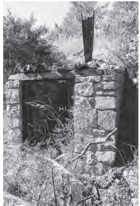
Figure 85. Ruins of first Cap Magazine, 2002. Roof has partially collapsed. Note remains of wooden vent. View looking northwest.
