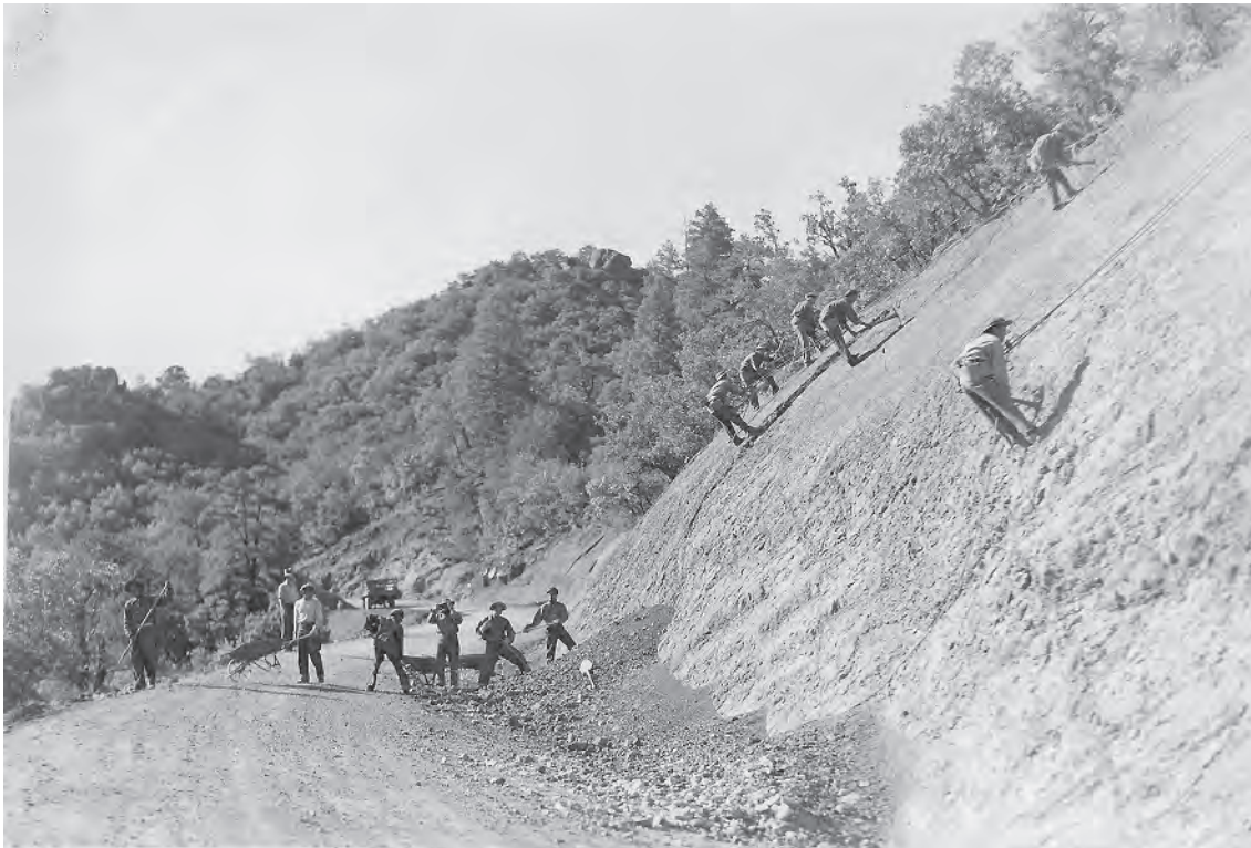
Figure 7. Road crew uses picks and shovels in backsloping effort on Bonita Canyon Highway.
