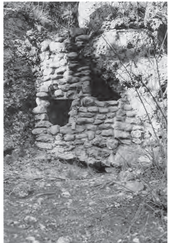
Figure 104. Remains of Cima Bear Cage built by CCC enrollees to house pet bear cub, 1993.
