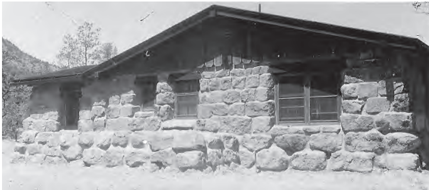
Figure 135. Basement entrance at rear of Residence #3, 1949. Note diminishing size of rock work from foundation up. View looking southwest.
