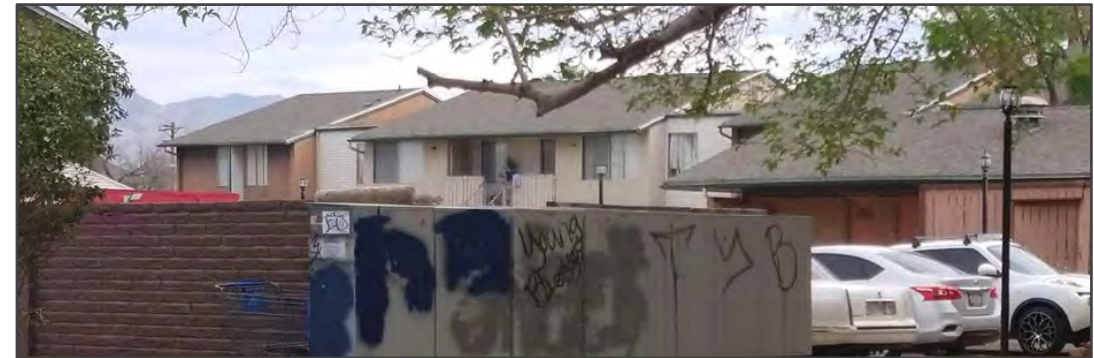
Figure 25. Graffiti and vandalism at community mailboxes.
