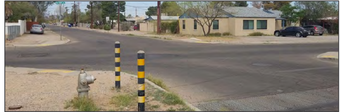
Figure 24. ADA-compliant ramps hindered by stormwater bollards at North Palo Verde Avenue and East Flower Street.
