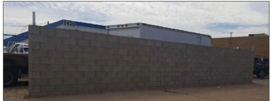
Figure 32. Underutilized vacant wall along East Grant Road.
